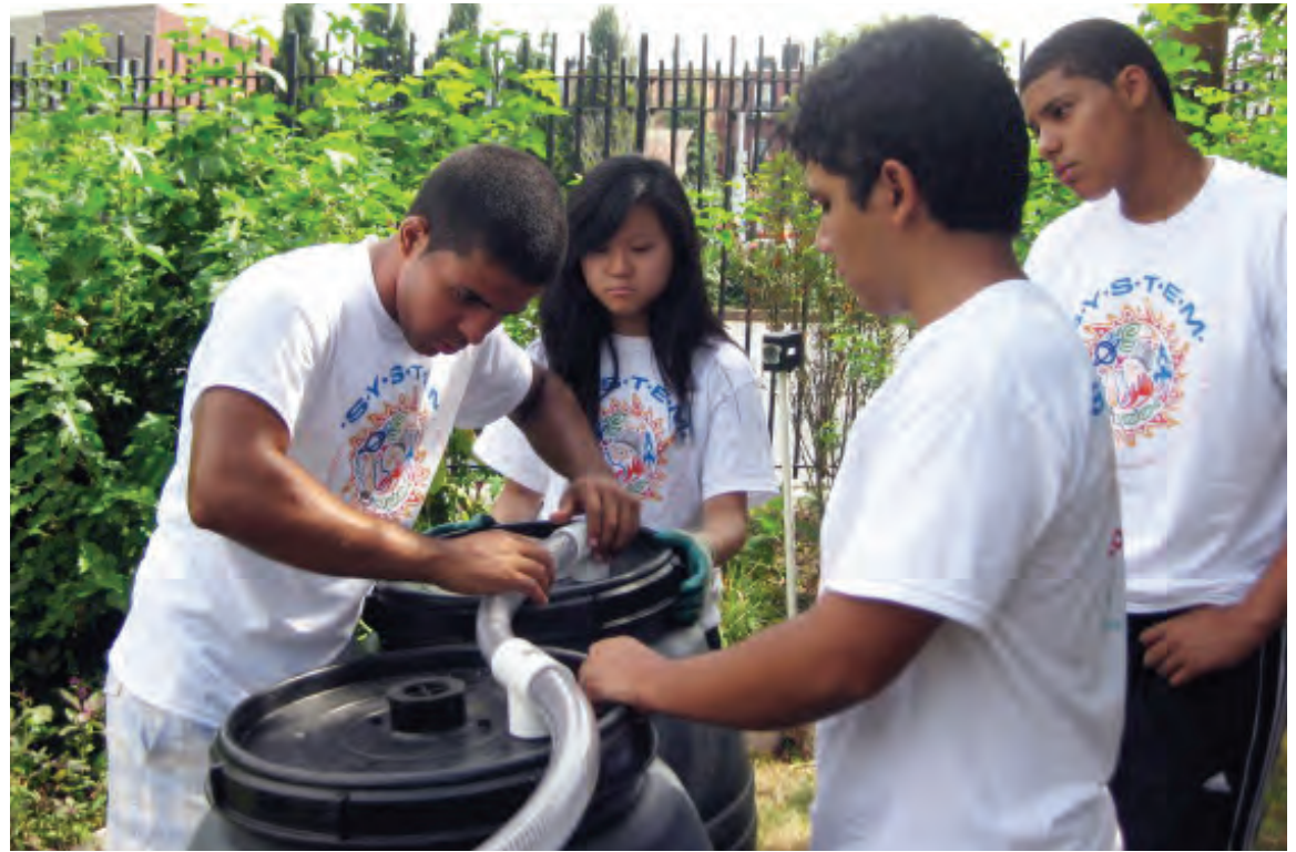
SYSTEM students construct the rain barrel catchment system in Lentol Garden. (Left to right): Kevin Negron, Erica Lei, Rai Munoz, and Donatello Meltz DeMeo.
